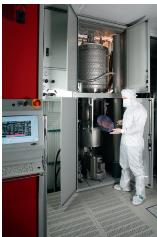
Fig. 1: Installation des PEDBAR-Vertikalofens im Reinraum des Fraunhofer IISB; The PEDBAR vertical furnace installed in the cleanroom of the Fraunhofer IISB.
